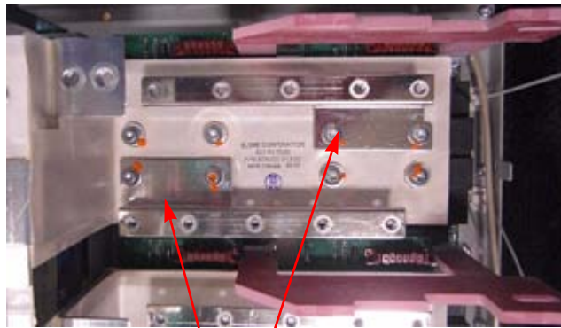
Inverter Snubber Brackets
